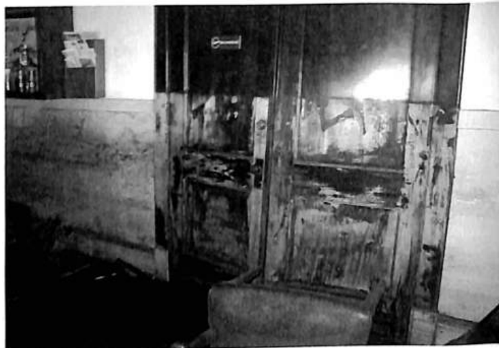
Sokol Cedar Rapids - Flood Line on Gym Doors
