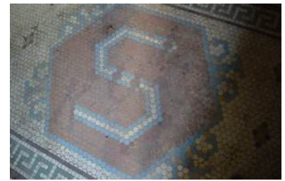
Though inundated with floodwaters in 2008, original tiles in the Sokol building in downtown Cedar Rapids survived. (photo/Cindy Hadish)
